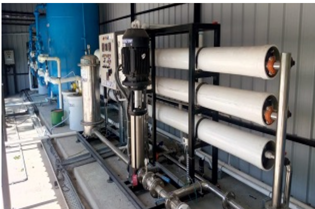
Reverse-osmosis plant installed in Chennai
